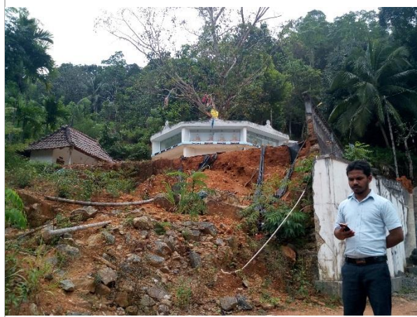
Fig b: Collapsed wall around the Boodhiya.
