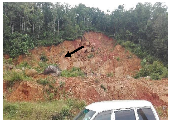
Fig b: The water supply line crossing the failed upslope
