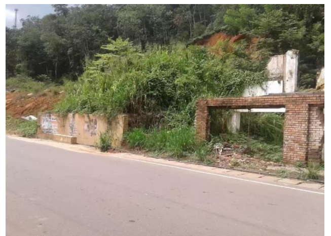
Fig d. Damage buildings located at up slope area
