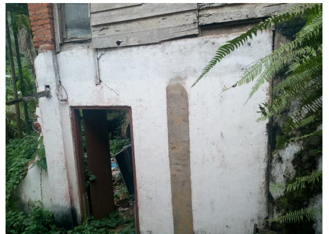
Fig f: Damage building located at down slope area
