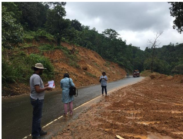
Fig a: Upslope and down slope of the failed slope
