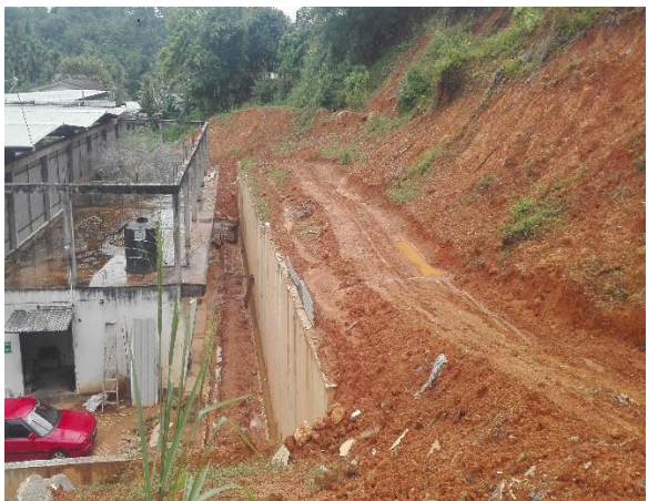
Fig e: Temporary road made by the owner of the filling station
