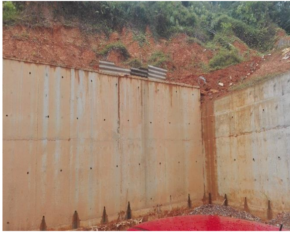
Fig a: Retaining wall made by Filling station owner right behind the filling station.
