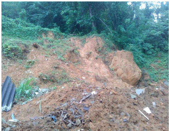
Fig c: Risky up slope area.
