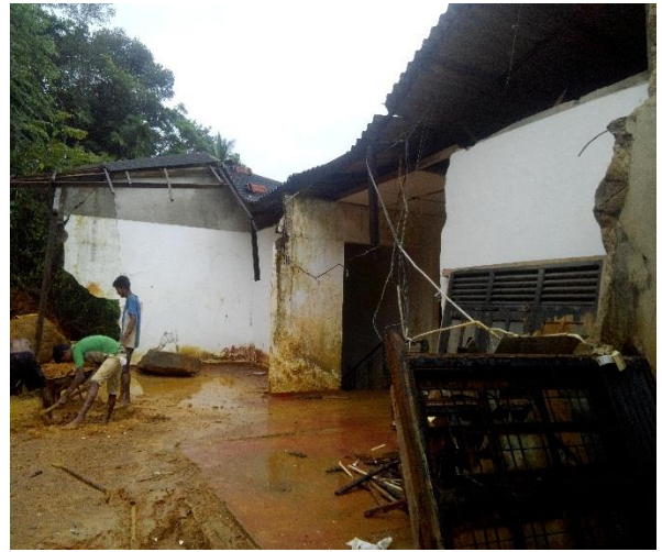
Fig 2b: A damaged house due to landslide
