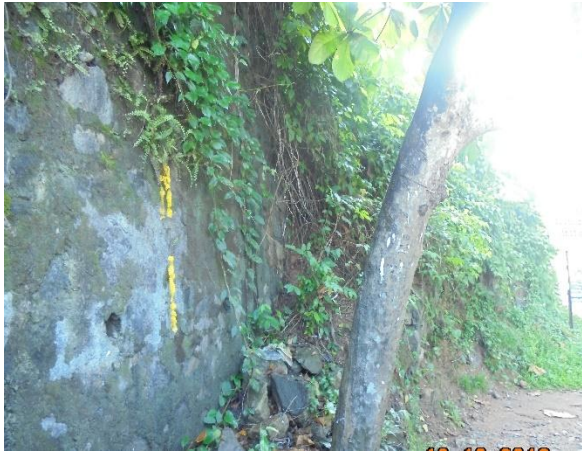
Fig 2c. Damaged retaining wall at the toe area
