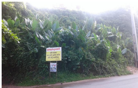
Fig 2a: upslope of the slope failure of the Kaluaggala Junction
