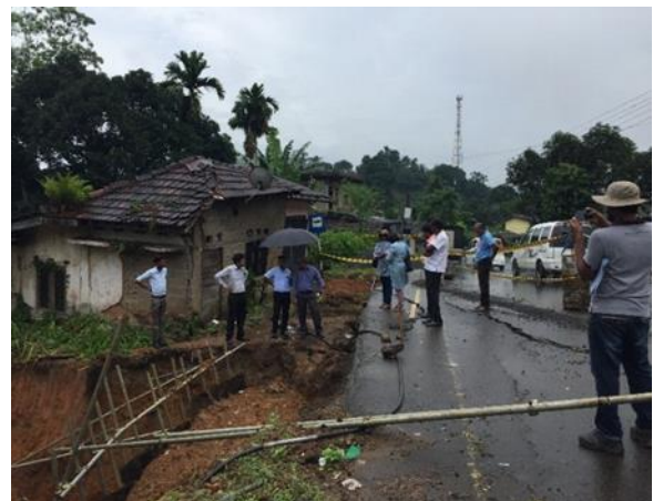
Fig f: Damaged road section at subsided downslope due to slope movement
