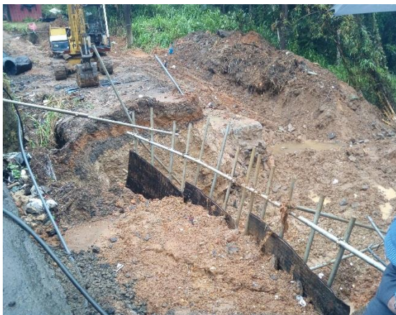
Fig e: Waterlines crossing the unstable section
