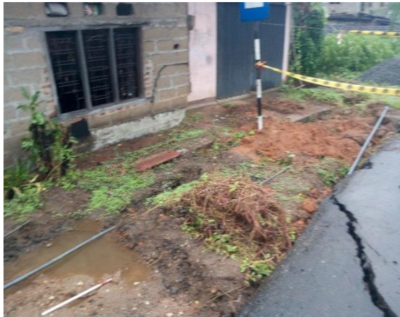
Fig c: Totally damaged house of – Mr Asnaka Chamara the house and the tension crack on the road
