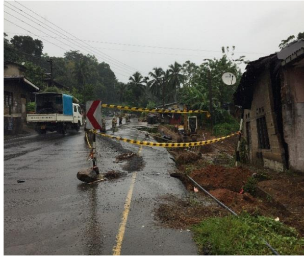
Fig 2a: Damaged road due to the creeping slope
