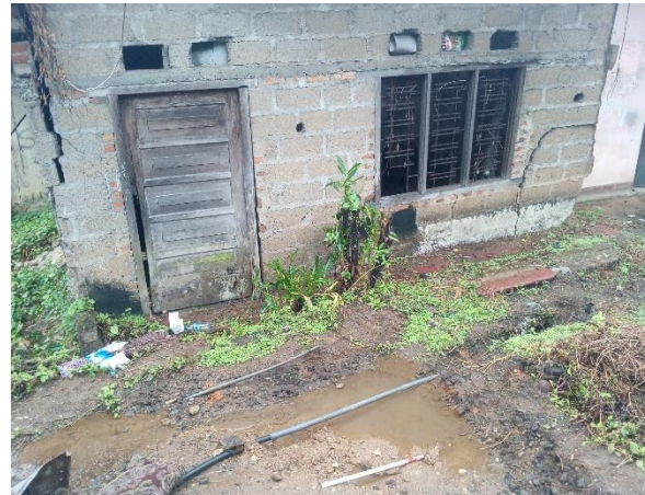
Fig d: Totally damaged house of Mr Asnaka Chamara
