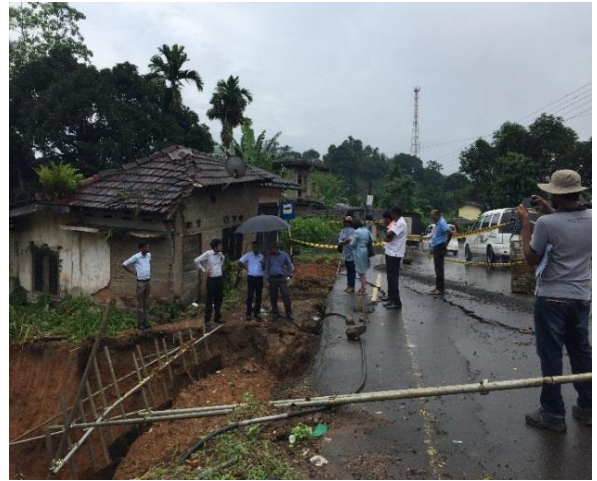
Fig 2d: Damaged road section and subsided downslope due to slope movement
