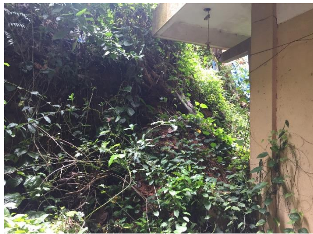
Fig 2c: Collapsed downslope area in the District Labour office
