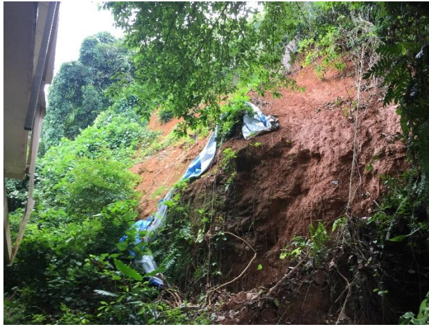
Fig 2a: The failed slope section of the North Western boundary of the Sri Sudharsanaramaya
