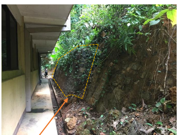
Fig 2d: Partially damaged retaining wall in the toe area
