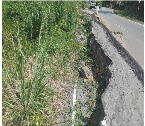
Fig 2b: Damaged road and Tension cracks on the road ( the dark color band)
