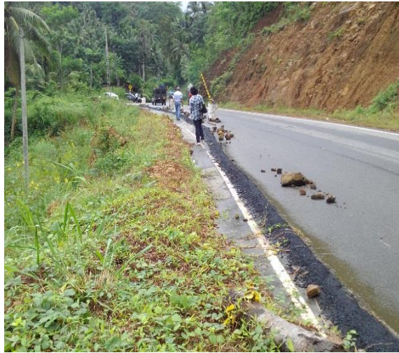
Fig a: A long tension crack on the road
