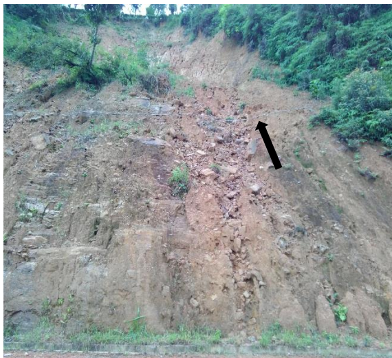
Fig c: The water supply line crossing the failed upslope.
