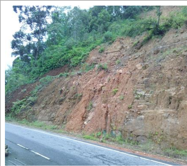
Fig 2a: The exposed surface of failed slope on the upslope
