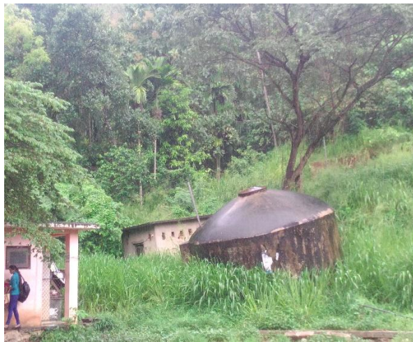
Fig 2c: Damaged water tank and building behind the water tank
