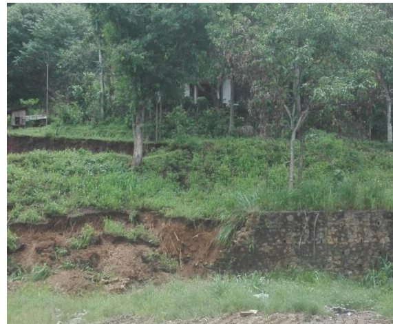
Fig f: Damaged retaining wall
