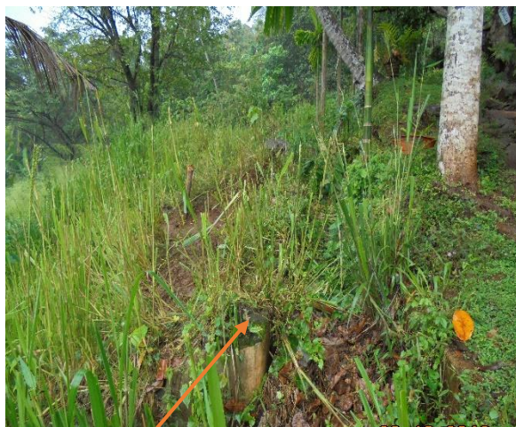
Fig e : Existing drainage system filled with mud and debris(Constructed in 1982)
