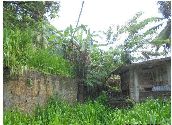
Fig d: Unstable retaining wall (Constructed in 1982)
