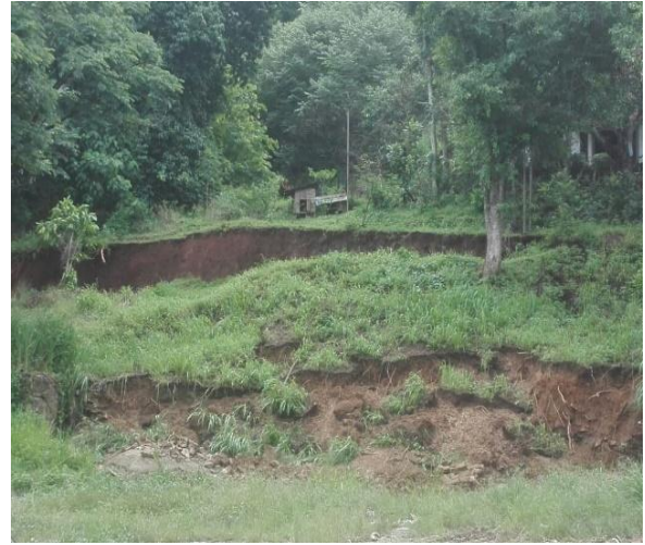
Fig 2b: Slope failure at the rear boundary of bus stand
