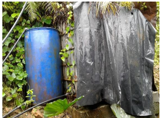
Fig 2f. Pipe lines directed to a water tank behind Gimanhala
