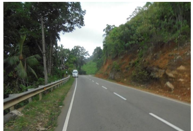
Fig 2b: Downslope of the road
