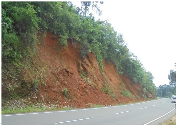
Fig 2a: Upslope of the road and slope failure
