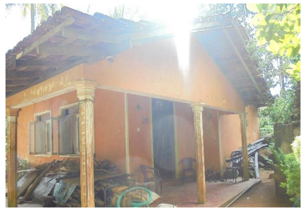
Fig 2c .A house identified as high risk
