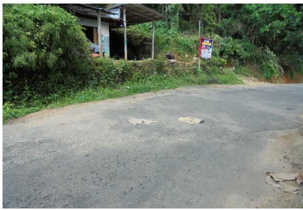
Fig 2c. Tension cracks on the road (RDA has covered the cracks by tar)
