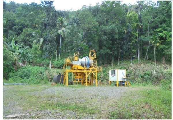
Fig 2b: DECMA Premix yard at the potential landslide area
