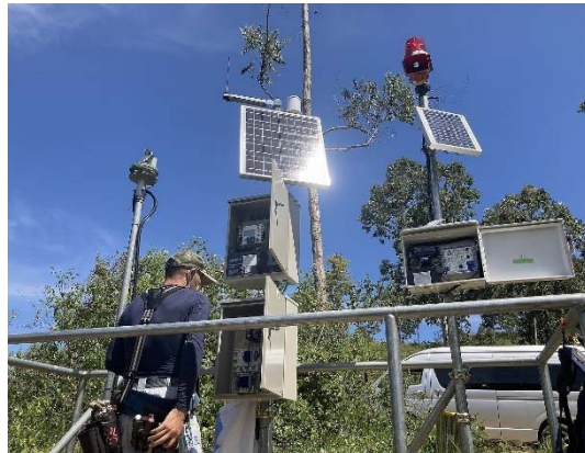
Installed landslide remote monitoring system in Weeriyapura, Badulla on January 25, 2022
