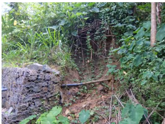
Photo 5.6 Collapse beside the horizontal drilling
