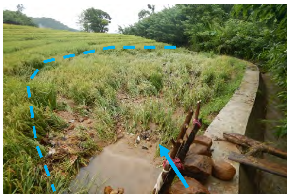
Photo 5.7 Stream Overflow from the Ditch
