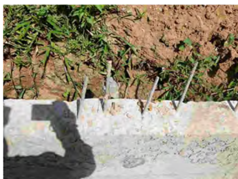
Reinforcing bars are not constantly placed
