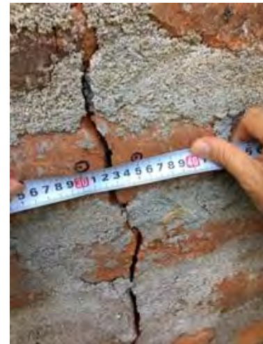
Figure 5.7 Cracks in May 2016
