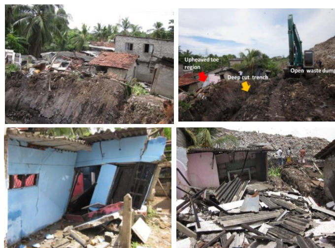
Figure 6: Ground movement and damages to houses due to deepening of the drainage canal; which removed toe support in the toe region at the South-West section in Oct 2012: Source: NBRO: 2013
